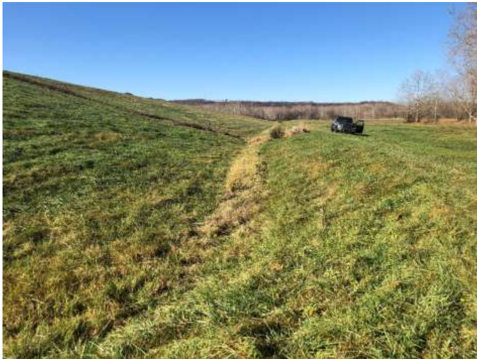
Photograph 39: North non-contact stormwater channel is clear of obstructions. North final cover lower slope is well vegetated and mowed annually. No evidence of animal burrows, erosion, or stability issues.
