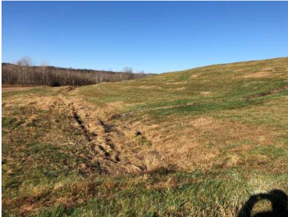
Photograph 23: South non-contact stormwater channel is clear of obstructions. South final cover lower slope is well vegetated and mowed annually. No evidence of animal burrows, erosion, or stability issues.
