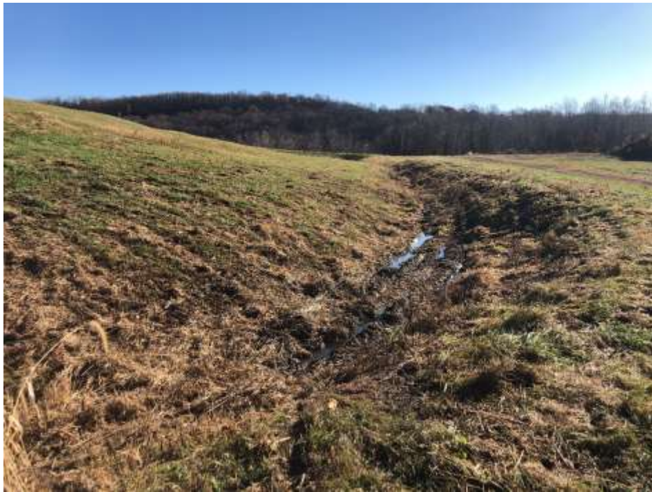
Photograph 25: South non-contact stormwater channel is clear of obstructions. South final cover lower slope is well vegetated and mowed annually. No evidence of animal burrows, erosion, or stability issues.
