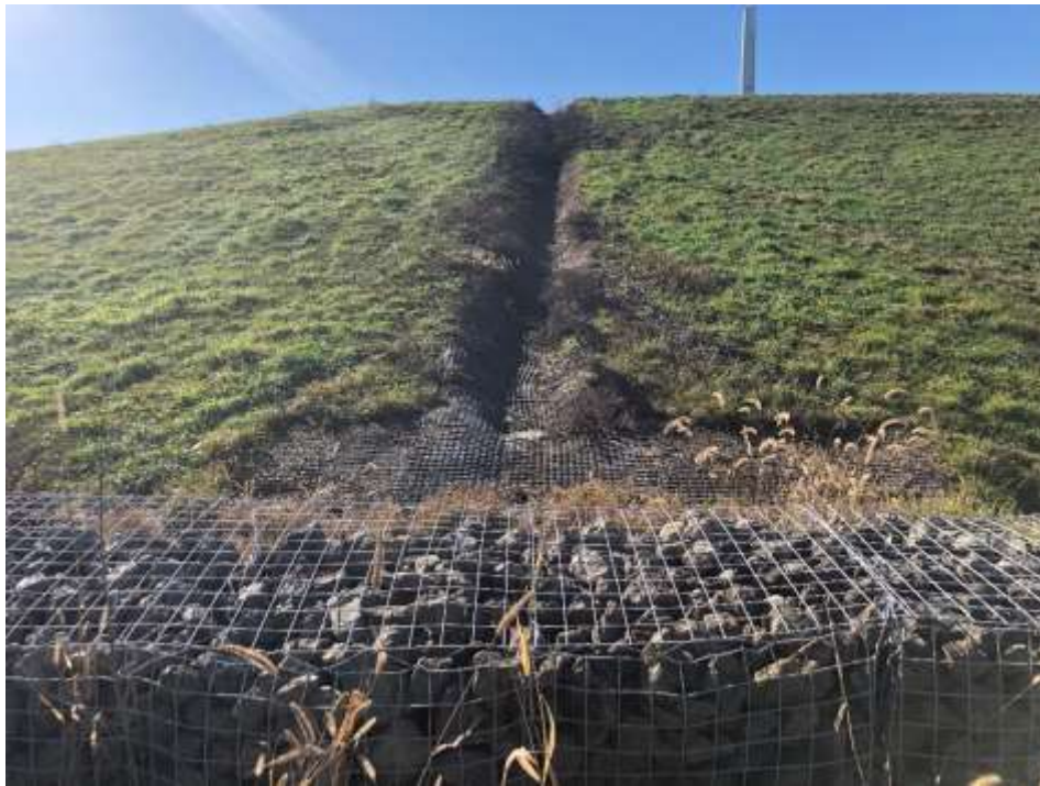
Photograph 37: Non-contact stormwater downchute is clear of obstructions. Gabion energy dissipator is installed at the junction with the stormwater (non-contact water) perimeter ditch.
