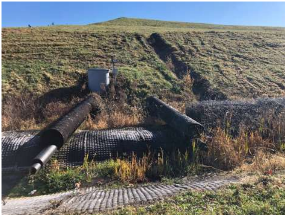
Photograph 30: Leachate collection zone and leak detection zone discharge pipes.
