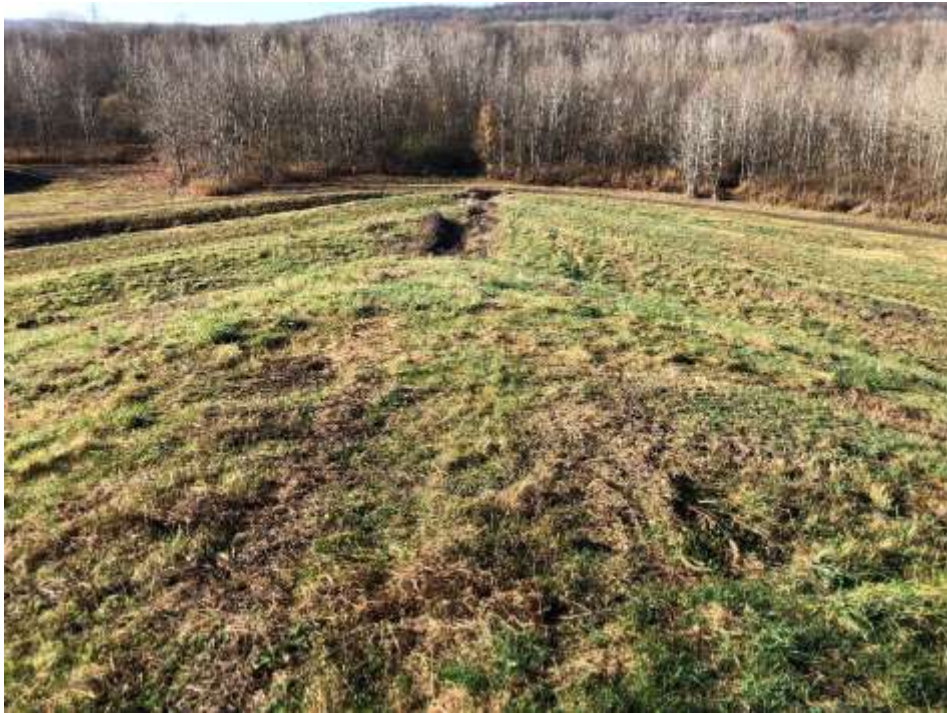
Photograph 11: Stage 4 southwest corner slope is well vegetated and mowed annually. No evidence of animal burrows, erosion, or stability issues.
