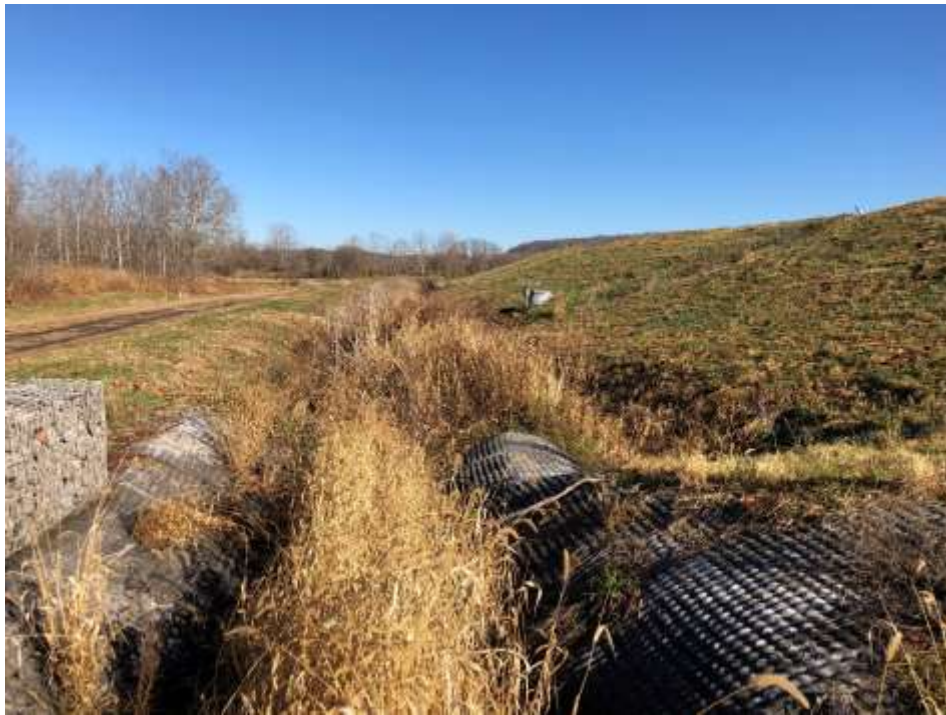
Photograph 29: West non-contact stormwater channel is clear of obstructions. West final cover lower slope is well vegetated and mowed annually. No evidence of animal burrows, erosion, or stability issues.
