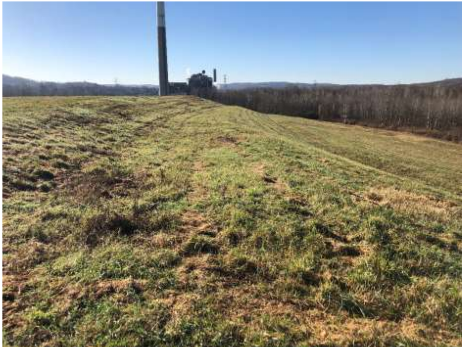
Photograph 8: Stage 4 west slope is well vegetated and mowed annually. No evidence of animal burrows, erosion, or stability issues.
