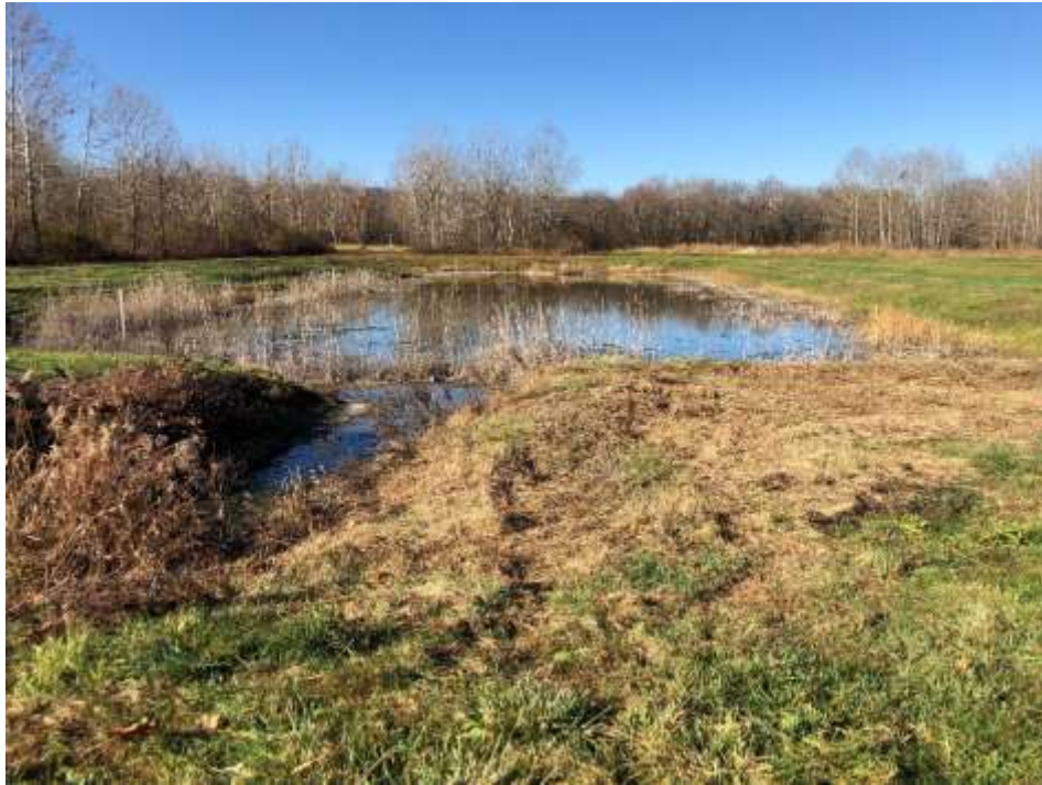
Photograph 33: Leachate (contact water) Pond. No evidence of animal burrows or liner damage.
