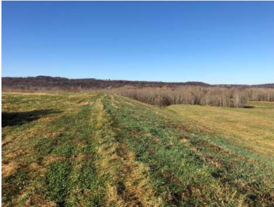
Photograph 5: Stage 4 north slope is well vegetated and mowed annually. No evidence of animal burrows, erosion, or stability issues.
