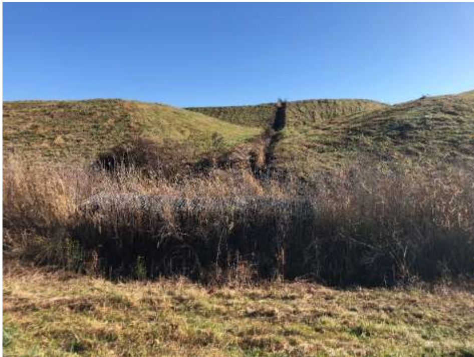
Photograph 31: Non-contact stormwater downchute is clear of obstructions. Gabion energy dissipator is installed at the junction with the stormwater perimeter ditch.
