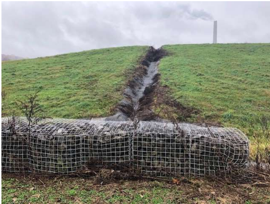
Photograph 15: Non-contact stormwater downchute is clear of obstructions. Gabion energy dissipator is installed at the junction with the stormwater (non- contact water) perimeter ditch.
