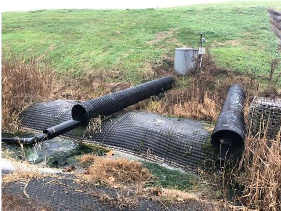
Photograph 7: Leachate collection zone and leak detection zone discharge pipes.
