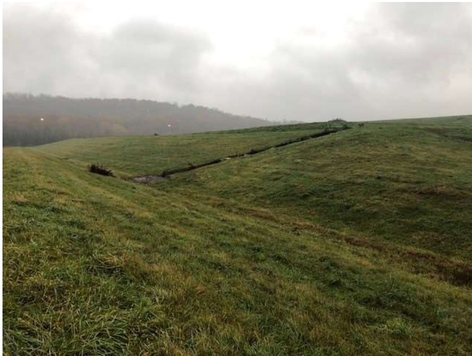
Photograph 13: North non-contact stormwater channel is clear of obstructions. North final cover lower slope is well vegetated and mowed annually. No evidence of animal burrows, erosion, or stability issues.
