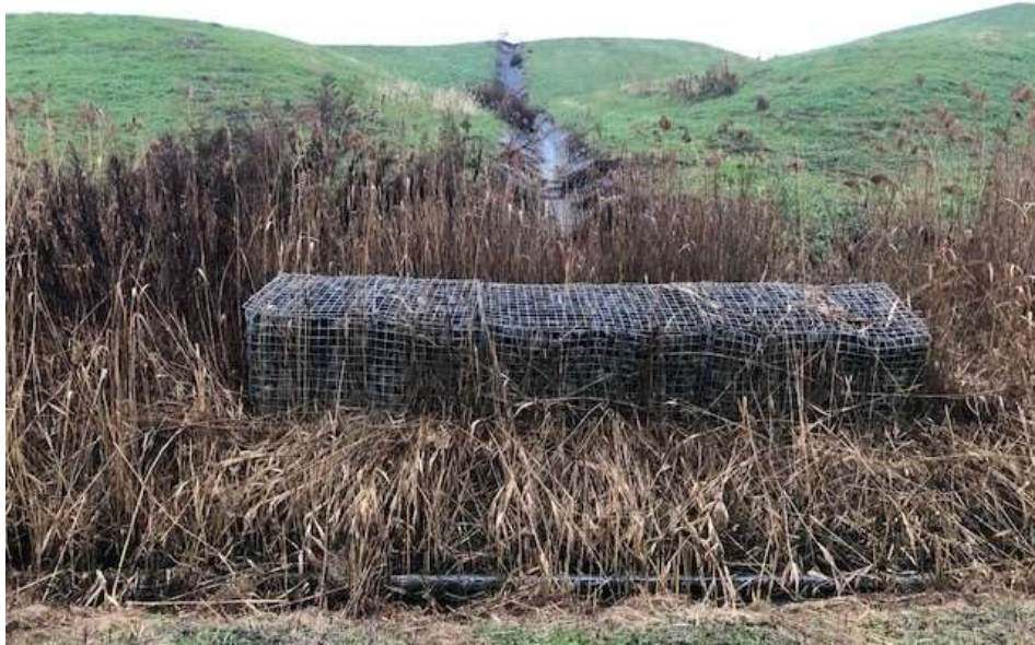
Photograph 9: Non-contact stormwater downchute is clear of obstructions. Gabion energy dissipator is installed at the junction with the stormwater (non- contact water) perimeter ditch.
