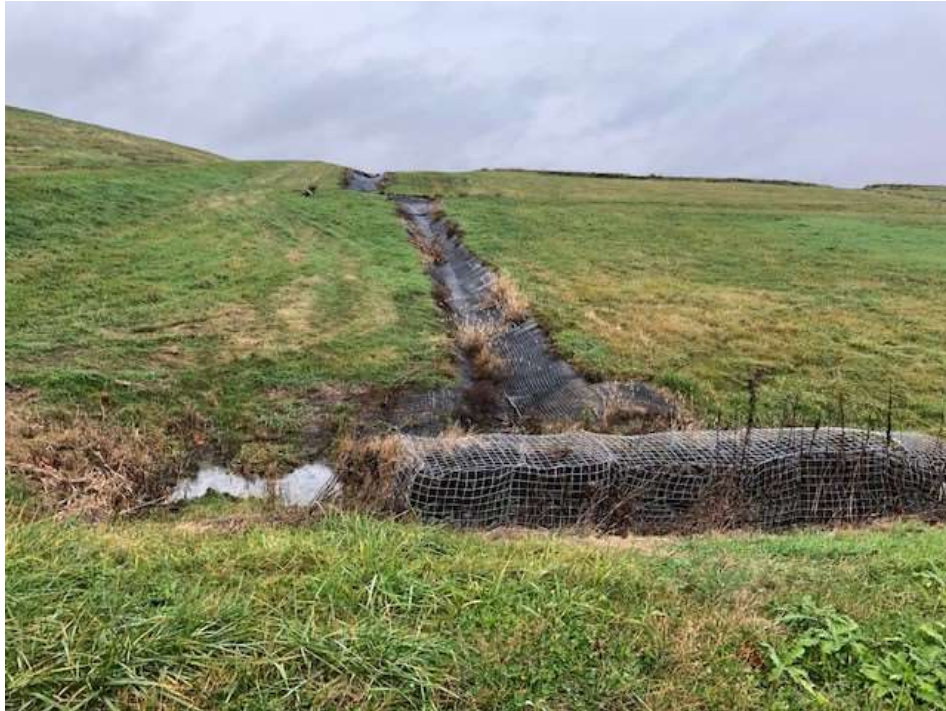
Photograph 25: Non-contact stormwater downchute is clear of obstructions. Gabion energy dissipator is installed at the junction with the stormwater (non- contact water) perimeter ditch.
