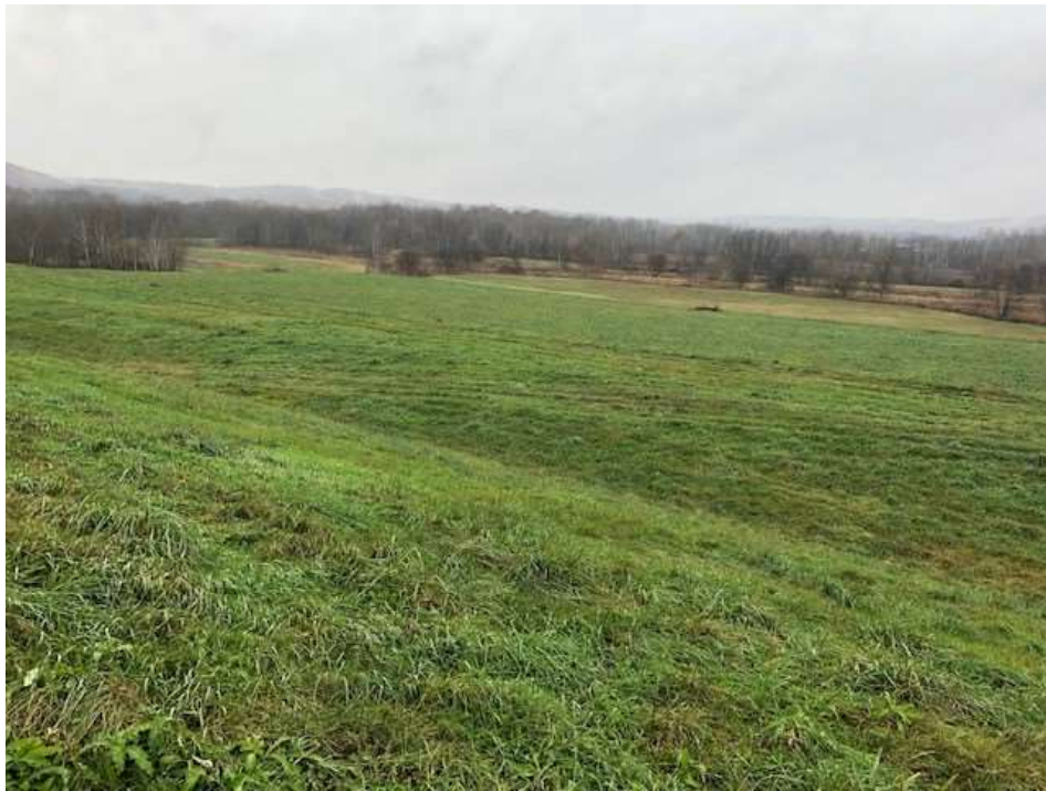
Photograph 29: Stage 5 final cover is well vegetated and mowed annually. No evidence of animal burrows, erosion, or stability issues.
