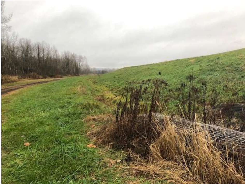
Photograph 5: West non-contact stormwater channel is clear of obstructions. West final cover lower slope is well vegetated and mowed annually. No evidence of animal burrows, erosion, or stability issues.
