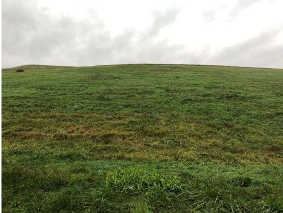
Photograph 23: Southeast corner final cover lower slope is well vegetated and mowed annually. No evidence of animal burrows, erosion, or stability issues.
