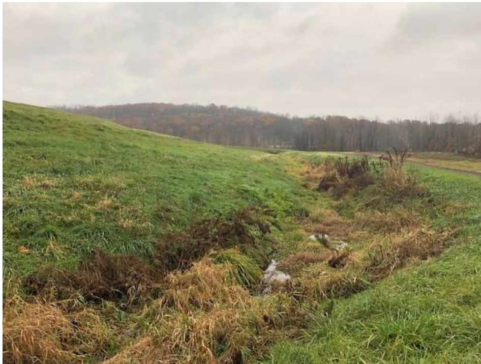
Photograph 3: South non-contact stormwater channel is clear of obstructions. South final cover lower slope is well vegetated and mowed annually. No evidence of animal burrows, erosion, or stability issues.
