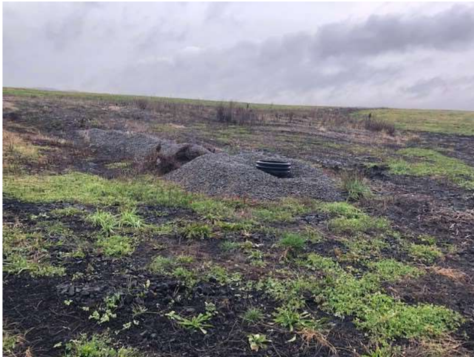
Photograph 36: Contact water collection riser in active area.
