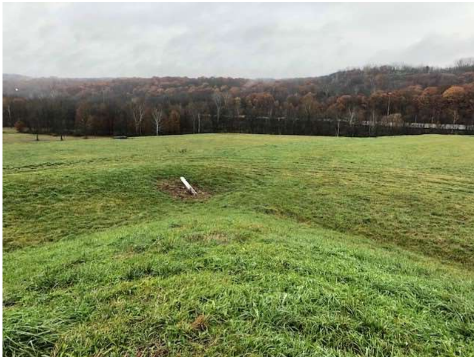
Photograph 28: Stage 5 final cover is well vegetated and mowed annually. No evidence of animal burrows, erosion, or stability issues.
