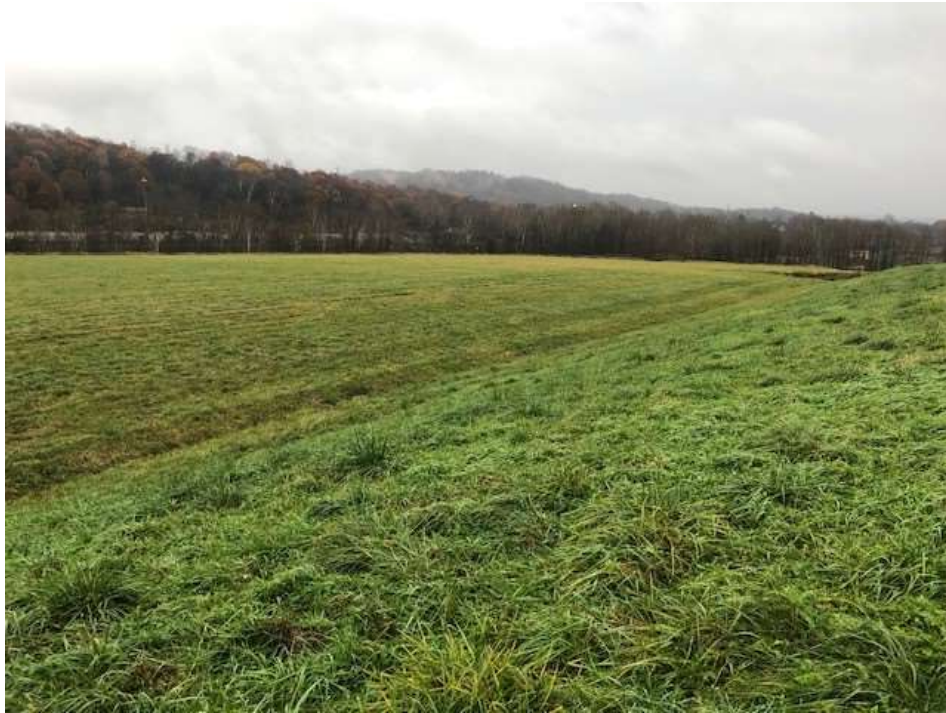
Photograph 27: Stage 6 final cover is well vegetated and mowed annually. No evidence of animal burrows, erosion, or stability issues.
