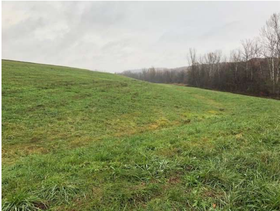
Photograph 21: East non-contact stormwater channel is clear of obstructions. East final cover lower slope is well vegetated and mowed annually. No evidence of animal burrows, erosion, or stability issues.
