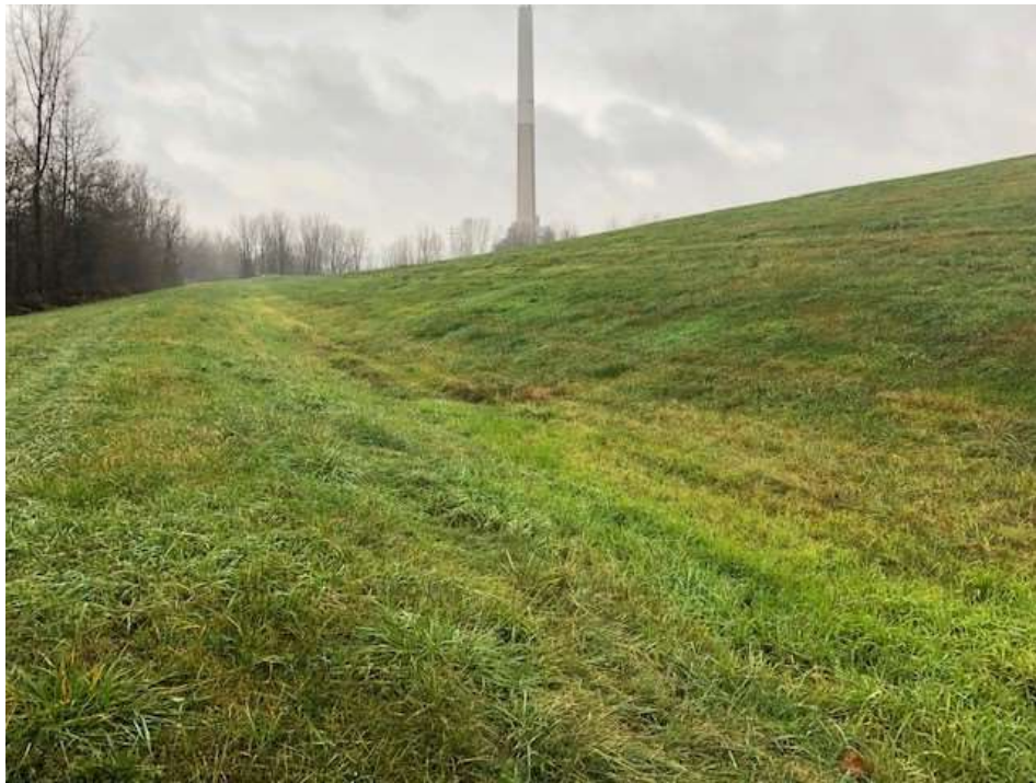
Photograph 19: East non-contact stormwater channel is clear of obstructions. East final cover lower slope is well vegetated and mowed annually. No evidence of animal burrows, erosion, or stability issues.
