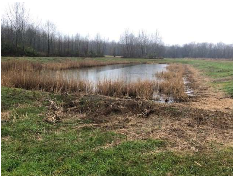
Photograph 10: Leachate (contact water) Pond. No evidence of animal burrows or liner damage.
