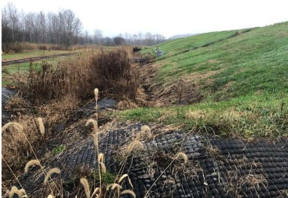
Photograph 8: West non-contact stormwater channel is clear of obstructions. West final cover lower slope is well vegetated and mowed annually. No evidence of animal burrows, erosion, or stability issues.
